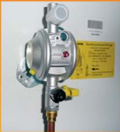
Typical Truma regulator installation mounted vertically. The 10mm copper compression fitting has been unscrewed for changing.
